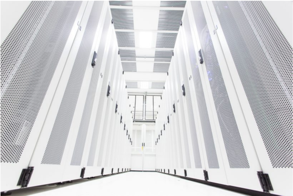
Server cabinets containing the data that is stored in the 'cloud'. Photo by A.R.E. Taylor.
