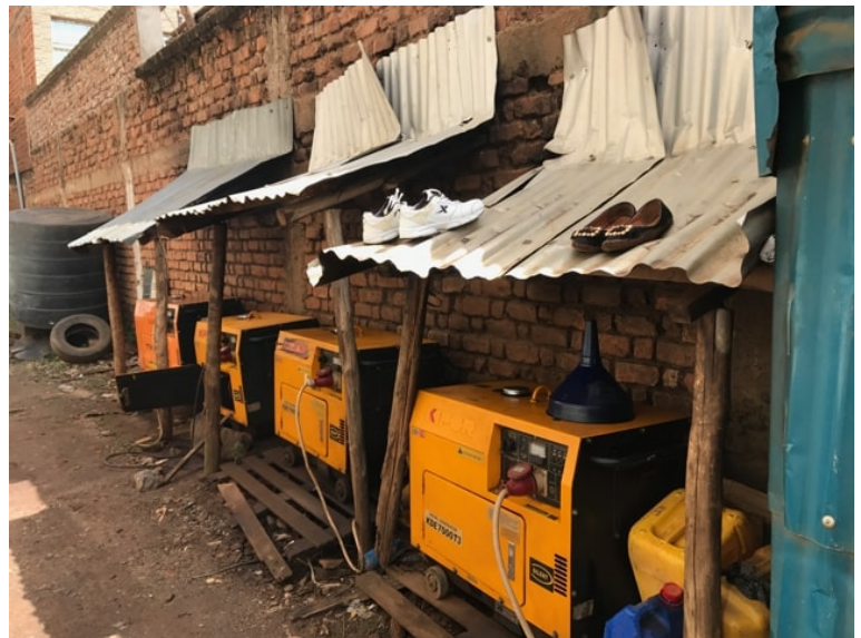
Generators in Bukavu, 2018
